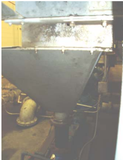
Figure 16-3 Discharge hopper arrangement on discharge side of GBTs.
