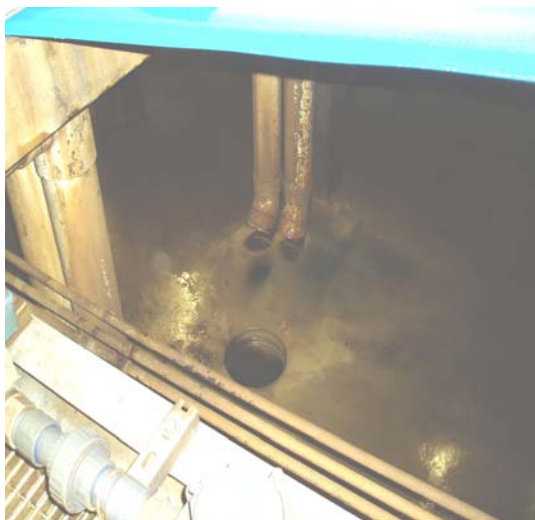
Figure 16-4 Gravity discharge of GBT filtrate.
