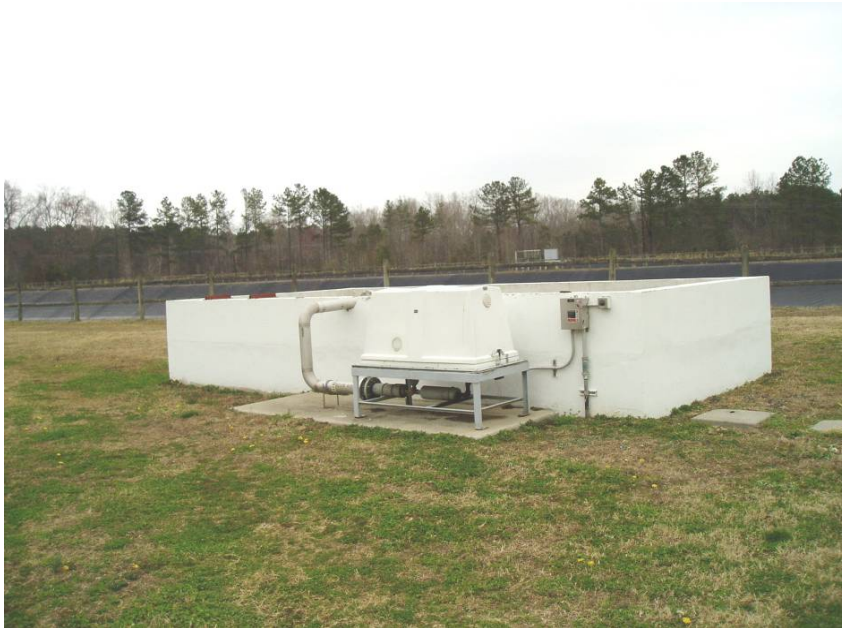
Figure 19-1: Scum Digester at South Cary WRF
